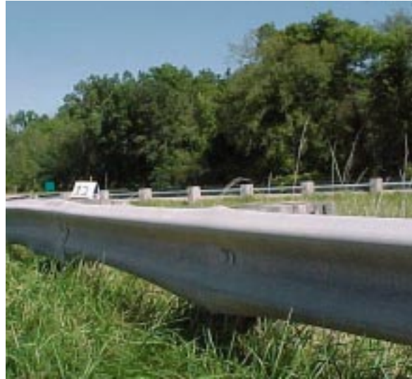
Figure 3. An example of minor guardrail damage.
