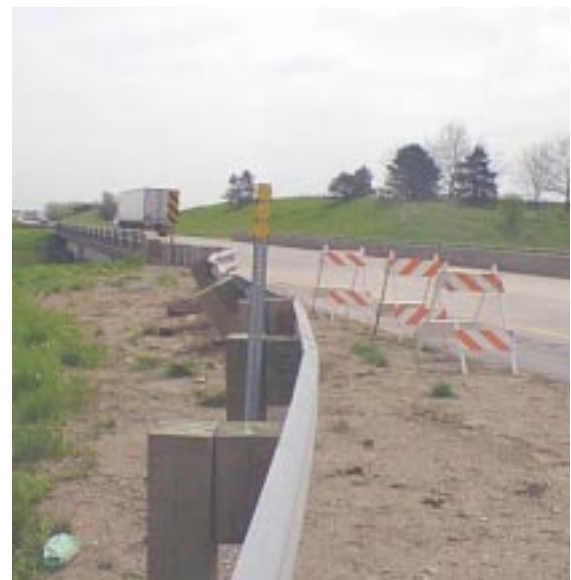
Figure 6. Bullnose damage (Case I98042701).
